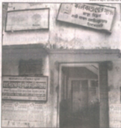
The dilapidated health centre at Hazi Mohd Square
